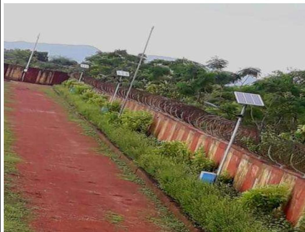
Installation of 125 no.s 50watt Solar Street light for plant area lighting and main road lighting
